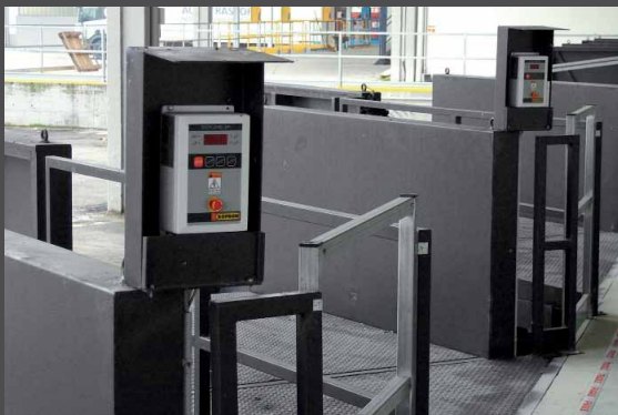
COLONNA PORTA QUADRO ELETTRICO CONTROL PANEL SUPPORTING POST
